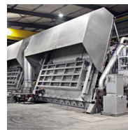
Casting furnace GO Holding and melting furnace
